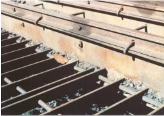
Figure 14 - Track Support Beam
