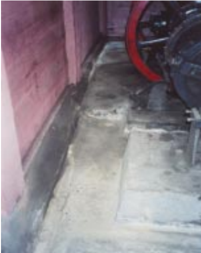
Figure 7 - Failed west bottom sill
